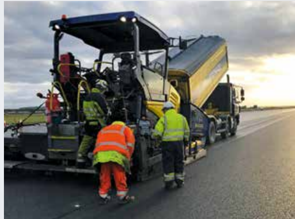
Above: Runway resurfacing at RAF Kinloss (courtesy of the Defence Industry Organisation)
